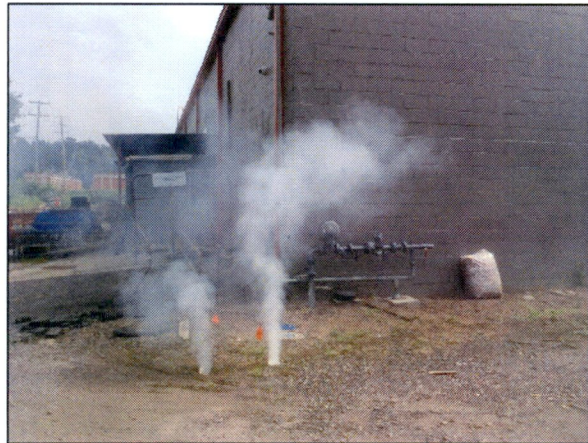
Missing and Defective Cleanout Line Segment (RV26) 8013-8012
