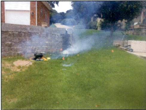
Smoke Testing Defect (RV26)8036-8032
