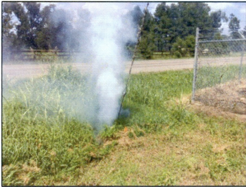
Mainline Defect (RV26)8043-8044
