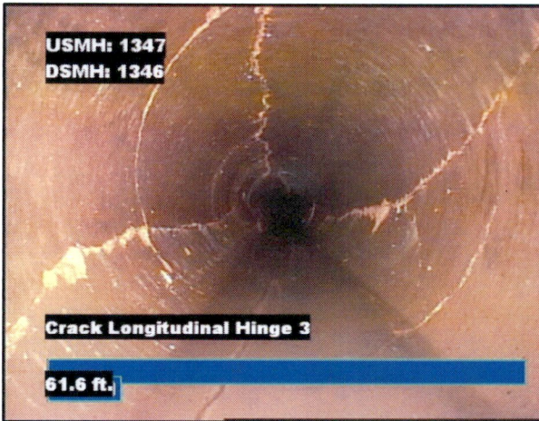
Hinge Cracks Line Segment 1347-1346
