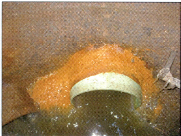
Defective Pipe Seal (RV26)8001
