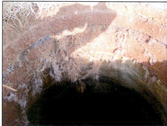
Defective Frame Seal (RV16)1420
