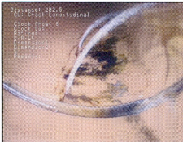
Active Infiltration Line Segment 1419-1417
