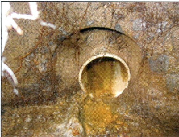
Defective Pipe Seal (RV26)8640
