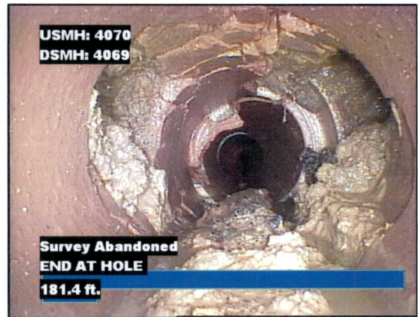
Hole with Void Visible Line Segment 4070-4069
