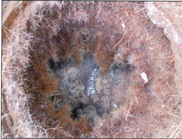
Manhole with Severe Roots (RV26)8632
