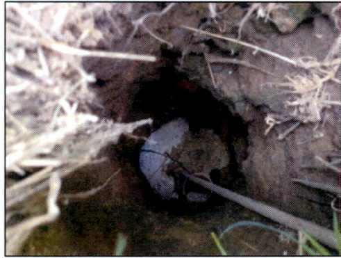
Mainline Defect (RV26)8043-8044
